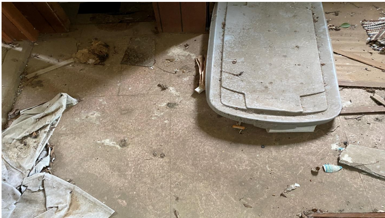
General of the asbestos floor tile located in the bathroom
