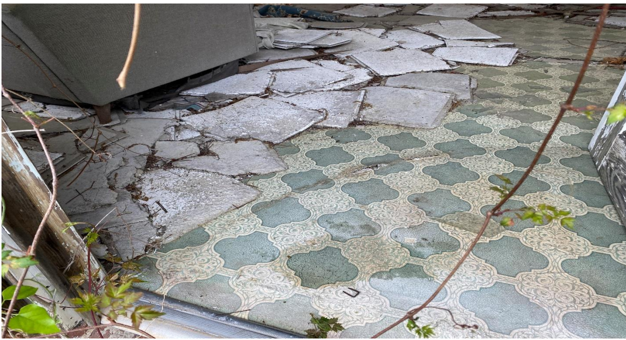
General of the asbestos flooring located in the patio area
