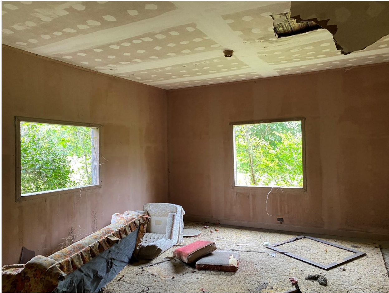
General view of the asbestos containing joint compound wll system located on the interior
